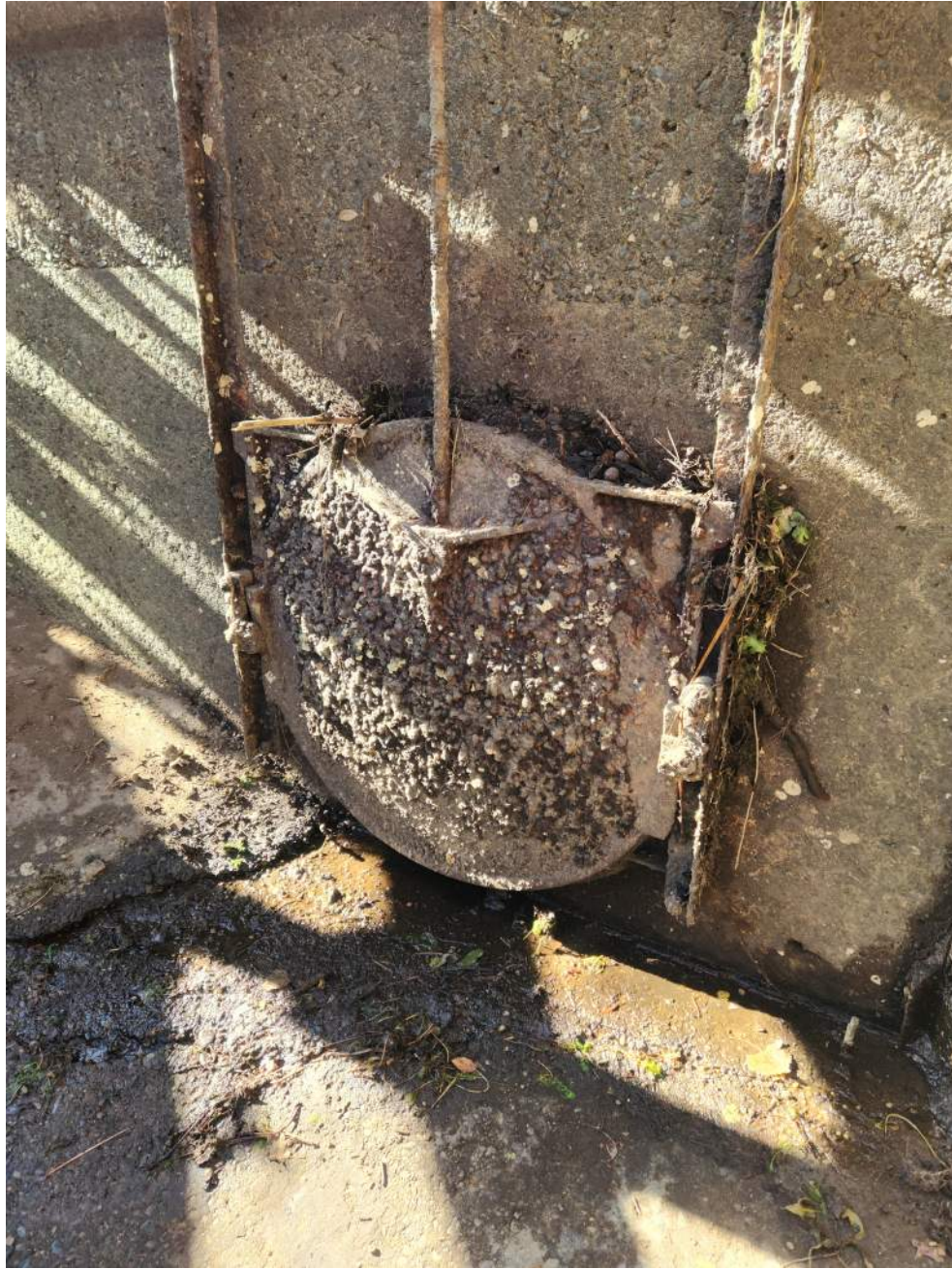
CIA Ditch gate to be removed and replaced
