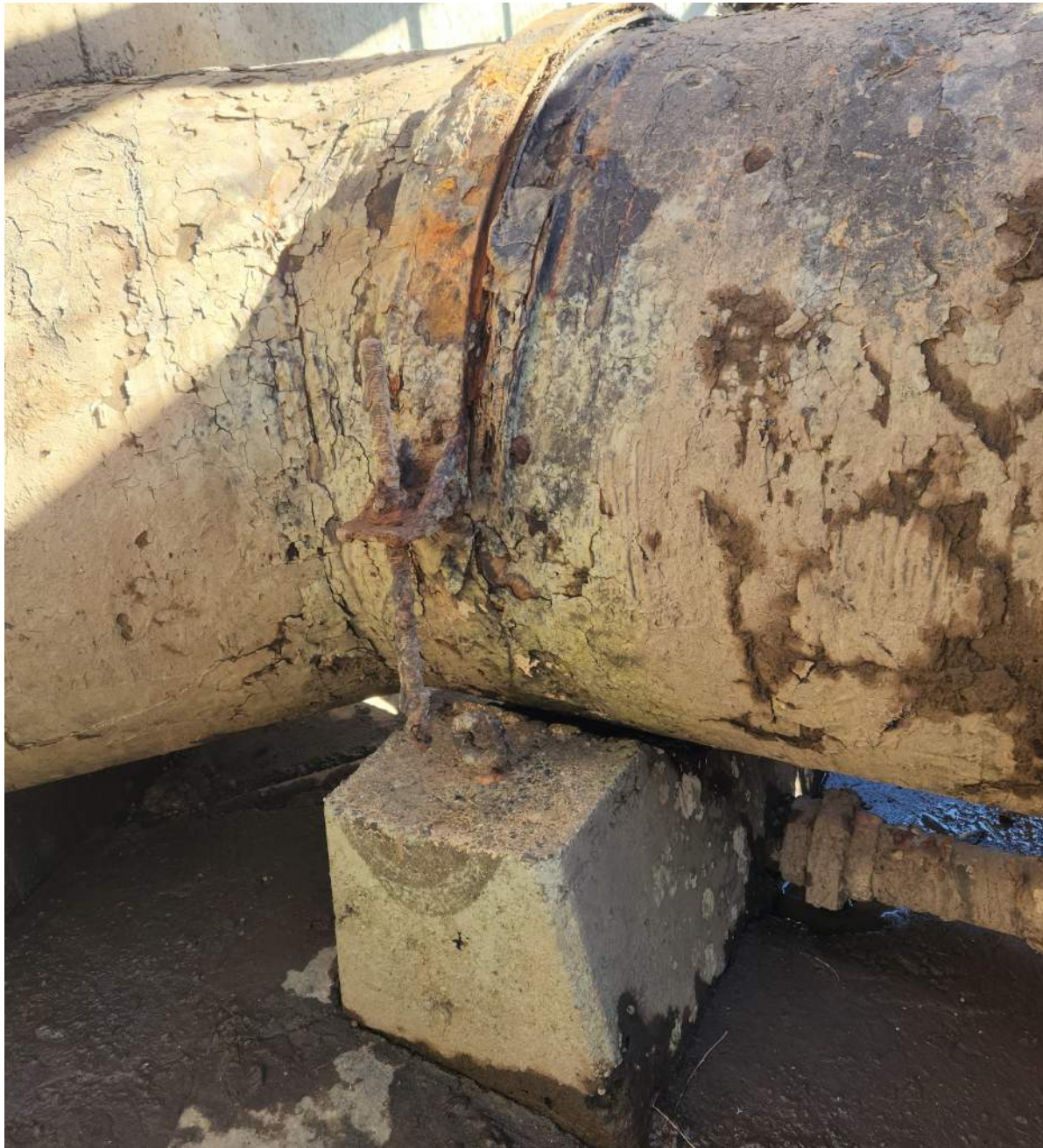
Pipe support to be repaired
