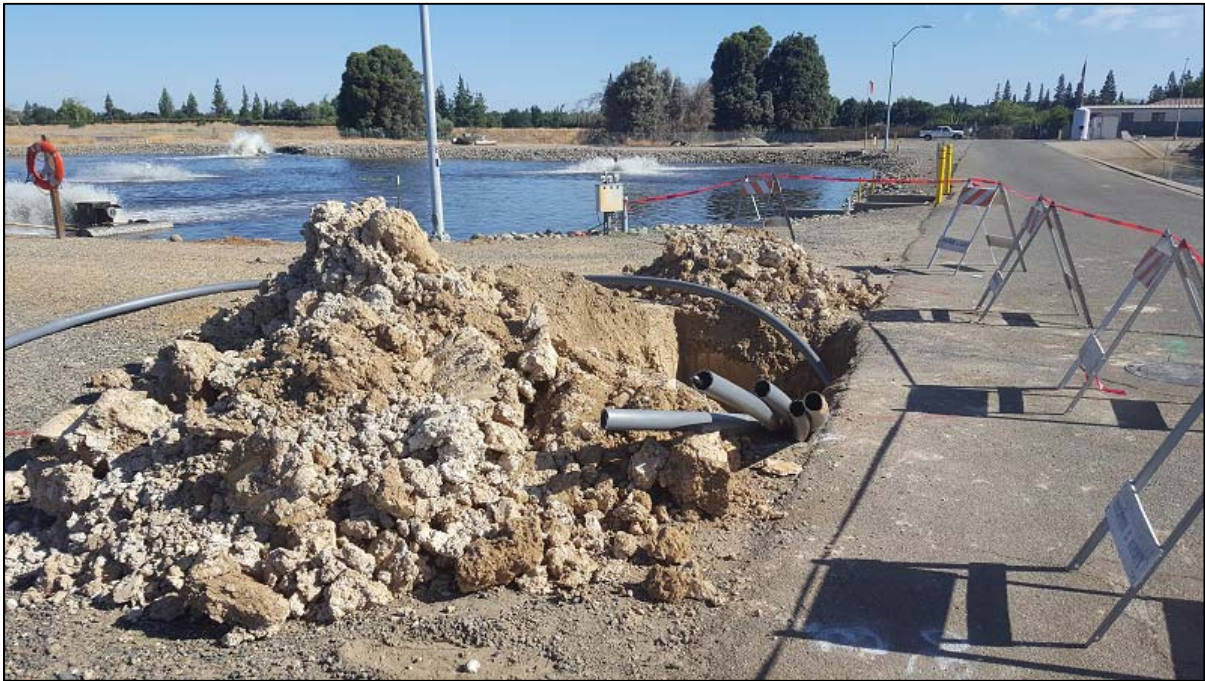
Photo of electrical conduits pulled through bore hole from PV site to Wastewater Plant.
